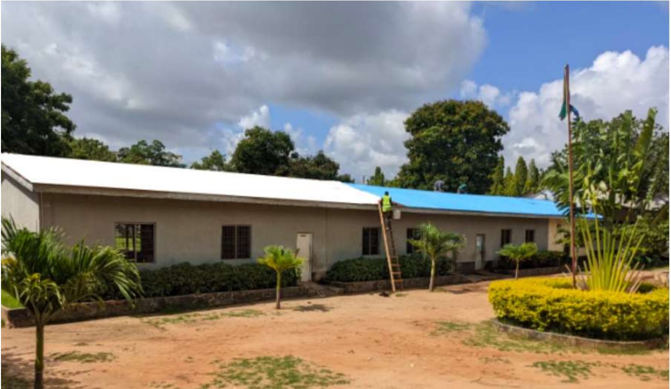
Figure 9. Example of a school roof painted with white paint. Image source: Proctor, J., 2022.
